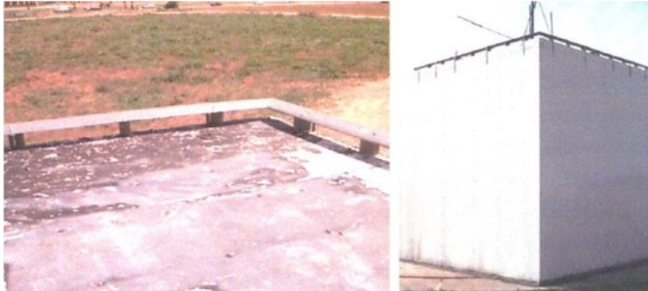
Figure 9. Roof-edge fairing on the TTU Building (after Banks, Sarkar, Wu and Meroney 2001).
